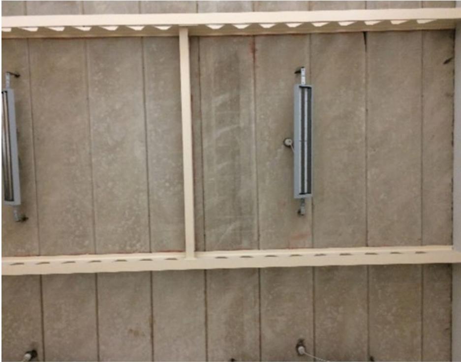
Figure 24: RAAC roof panels
