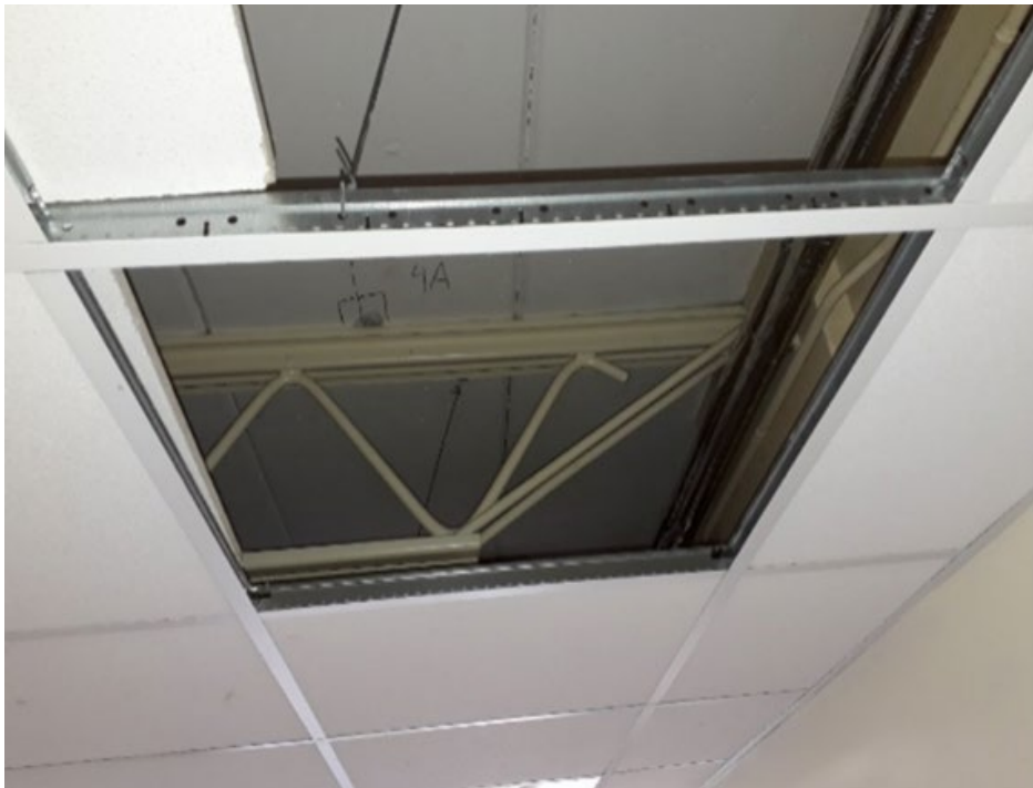
Figure 26: RAAC roof panels accessed through suspended ceiling
