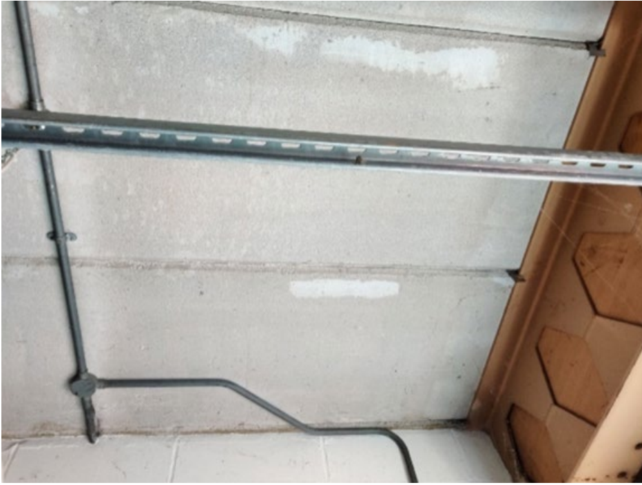
Figure 25: RAAC roof panels
