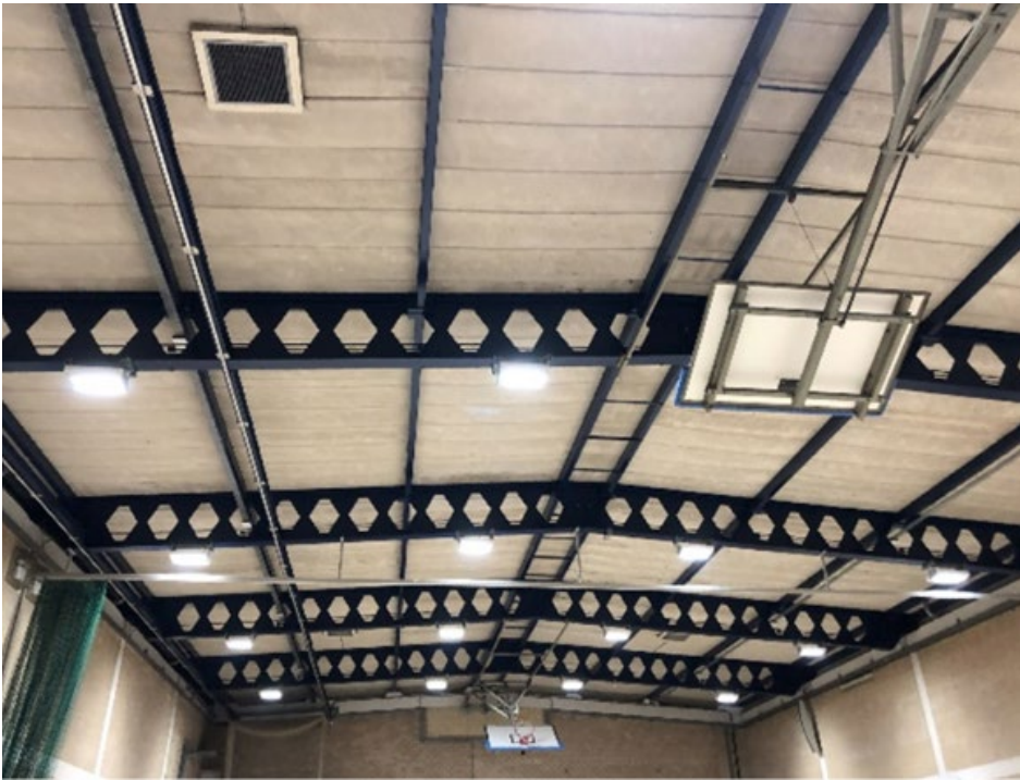
Figure 23: RAAC roof panels in sports hall
